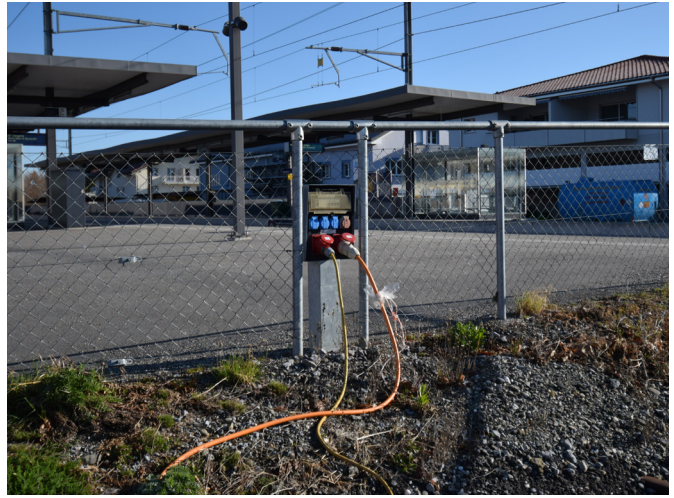
Power distribution box at Oberriet railway station
