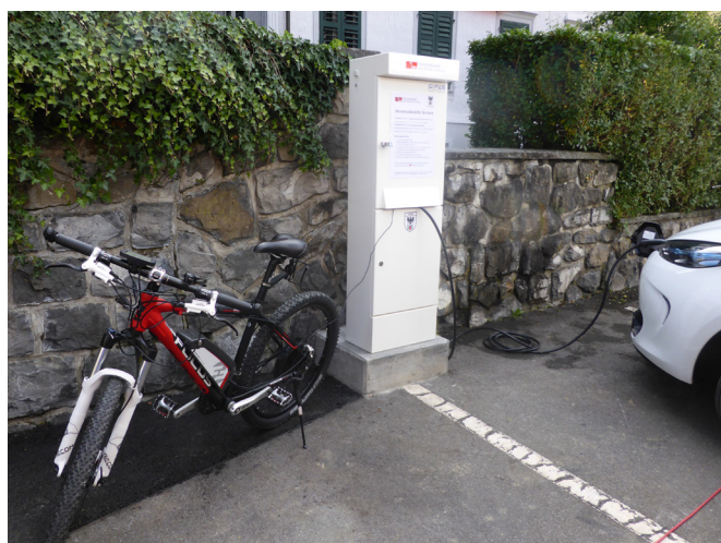
Electric vehicle charging station, electricity station EBS Schwyz
