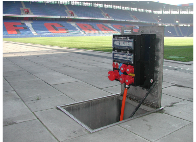
Underfloor distributor system, St.Jakob-Park stadium in Basel
