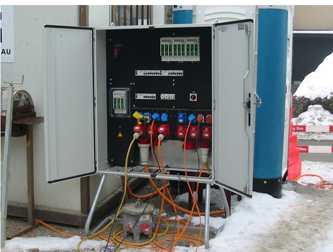
Main distributor on a construction site
